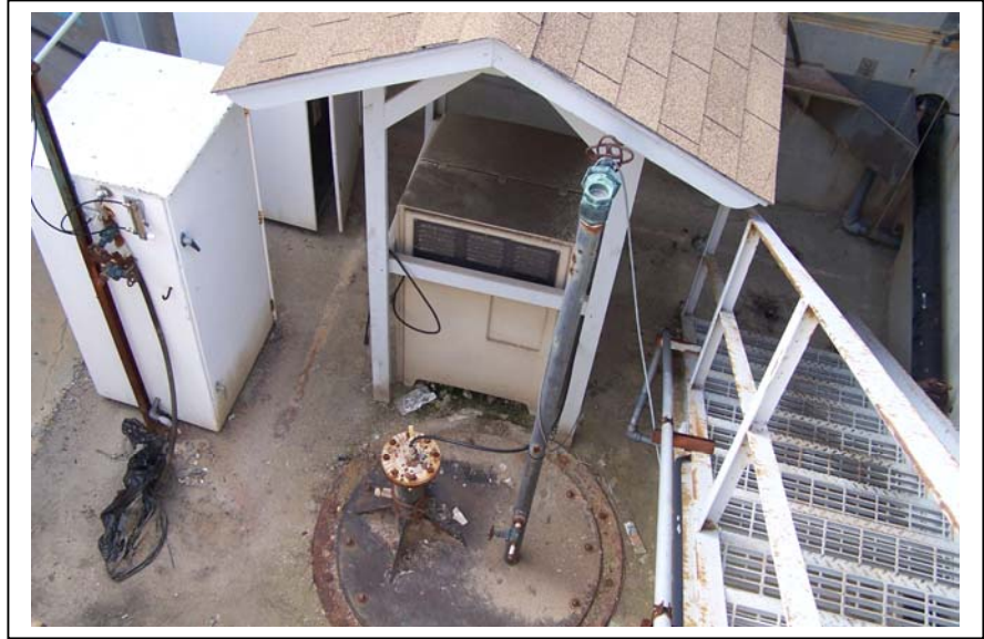
Divers will access the 5-mile outfall from this shaft located inside Hyperion.
